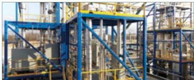
Woodland Biofuel's pilot plant in Sarnia, Ontario.
