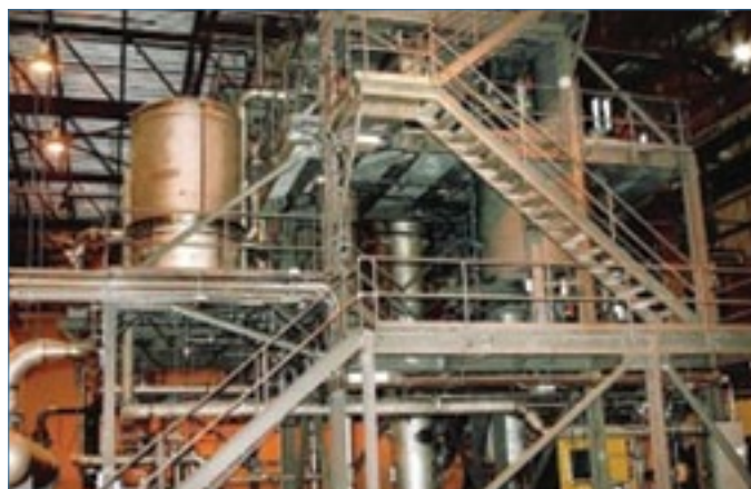
Inside Ensyn's Renfrew Rapid Thermal Processing plant.
