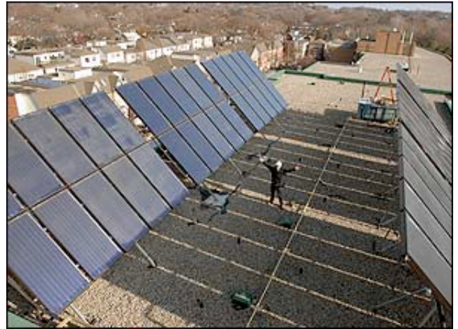
MICHAEL STUPARYK/TORONTO STAR Scale of project atop Coatsworth Ave. seniors residence is apparent as Alex Winch of Mondial Energy Inc., in his hard hat, stands between the rooftop installations of solar panels his company has had installed.
